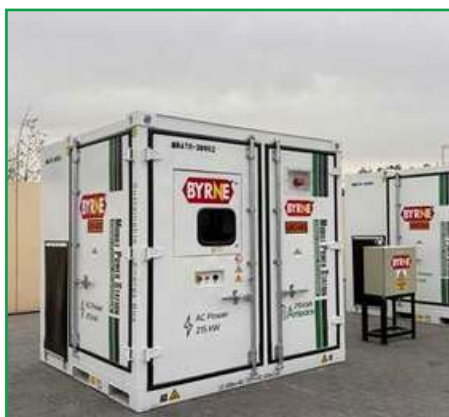
BEES (Battery Energy Storage Systems)
