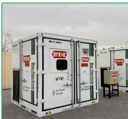
BESS (Battery Energy Storage Systems)
