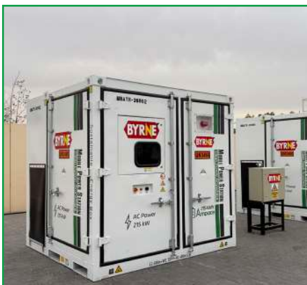
BESS (Battery Energy Storage Systems)
