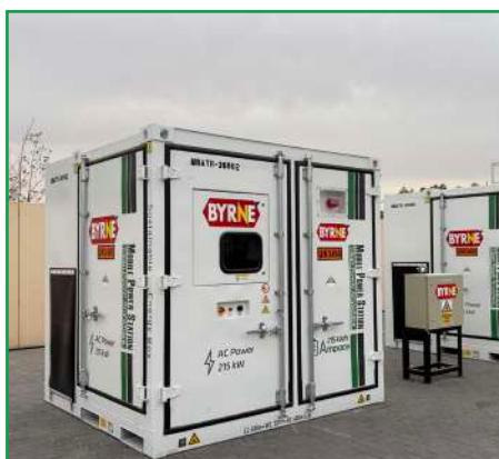
BESS (Battery Energy Storage Systems)
